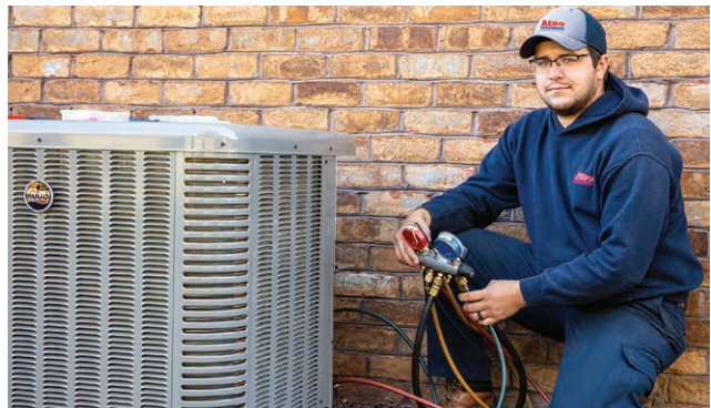
TUNED UP: An Aero Energy technician performs regular maintenance on an outdoor HVAC system to help improve its efficiency.
