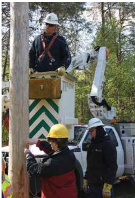
WORKING TOGETHER: Journeyman First Class Dan Leonard works from his bucket truck to attach the back-stop cable on a pole that will be used for an archery backdrop. Scout Achilles Light, bottom left, wraps the cable on a spool under the watchful eye of Journeyman First Class Tyler Miller.
