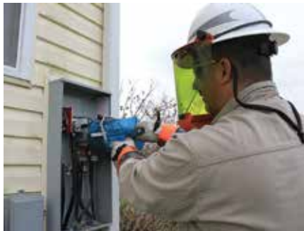
METER SAFETY: Line Serviceman Jon Fetter pulls the meter on the side of a member's residence so that additional work can be performed. Any time a meter is pulled, Adams requires that an employee of the cooperative perform the work.
